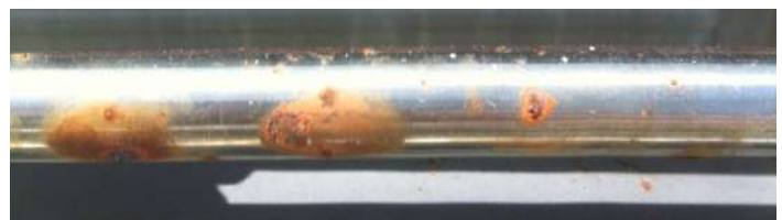
Corrosion from weld slag on 2507/UNS S32750 Super Duplex.
