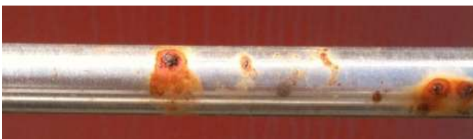
Corrosion from weld slag on 316L/UNS S31603 SS.
