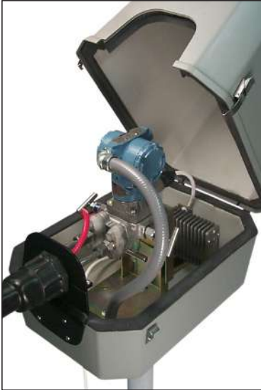
1. Traditional flange mounted instruments with vertical heater
